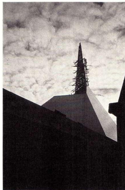
The new Estonian Methodist Church in Tallinn showing the limestone base and steeple under construction. Designed by Künnapu and Padrik Architects.
