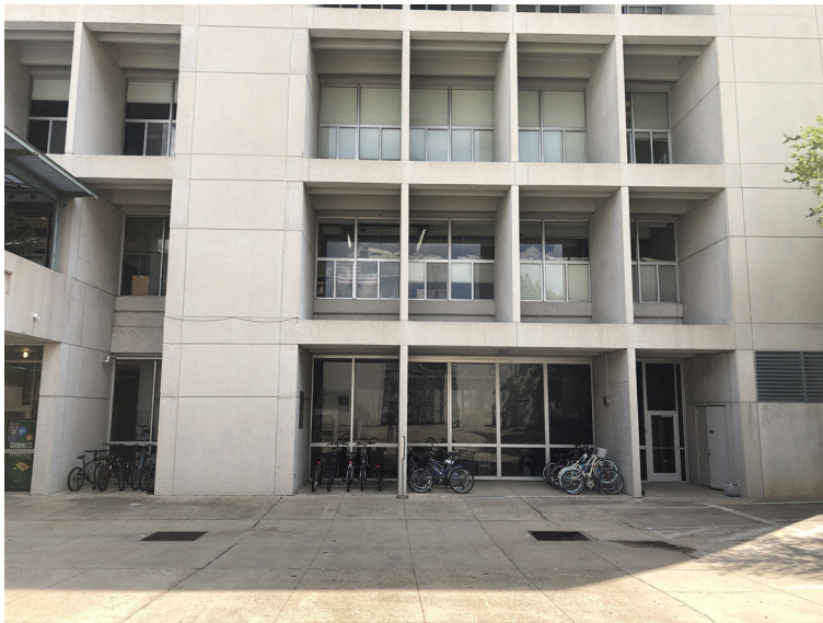
Figure 4 Langford Architecture Center A, north facade, showing the louvres or wall coffers to host the infill micro-housing
