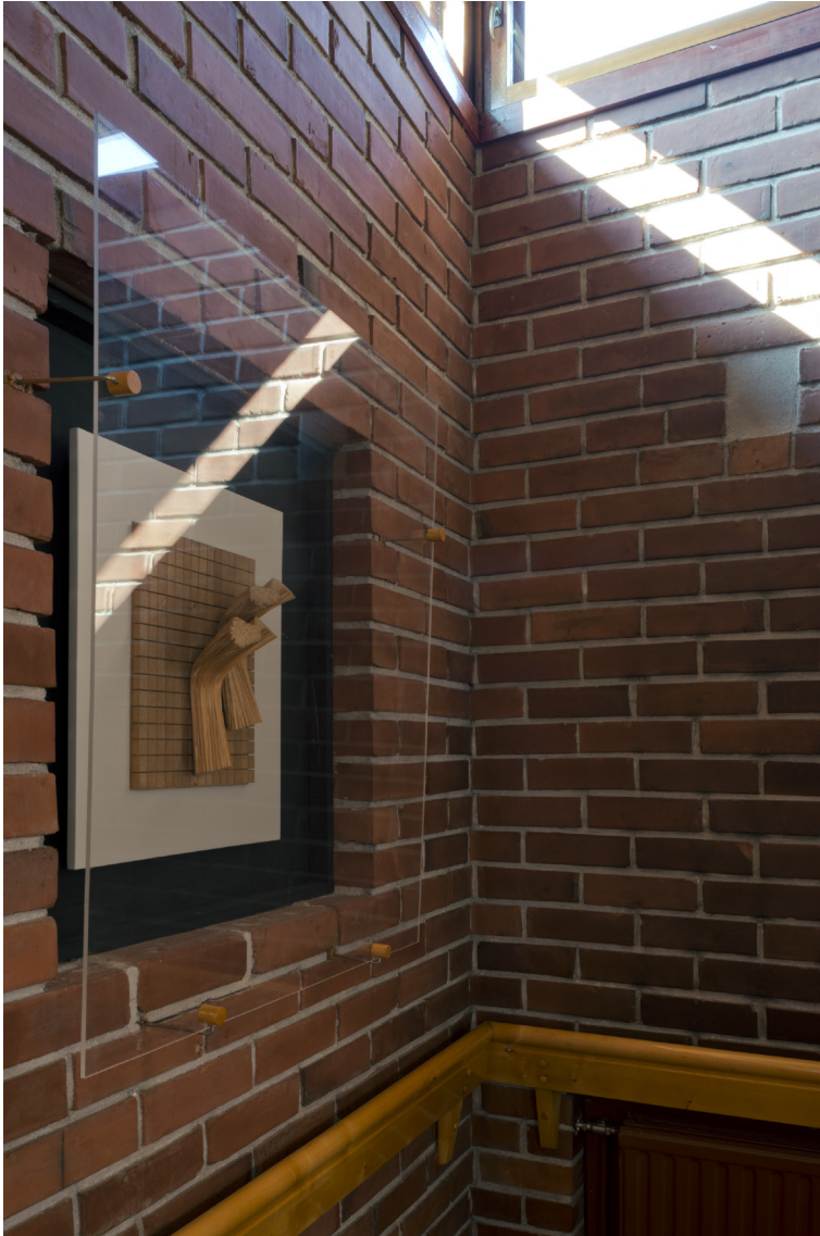
Picture 5 The landing with the relief in 2014; originally, there was the option of an additional window on the right (AAF digi2266 / Holma).
