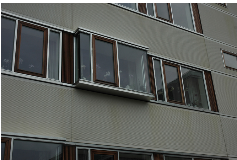
Figure 13 In connection with the renovation of Gyldenrisparken, new bay windows were installed in the kitchens. This greatly improved the view and daylight. Photo: Tegnestuen Vandkunsten.
