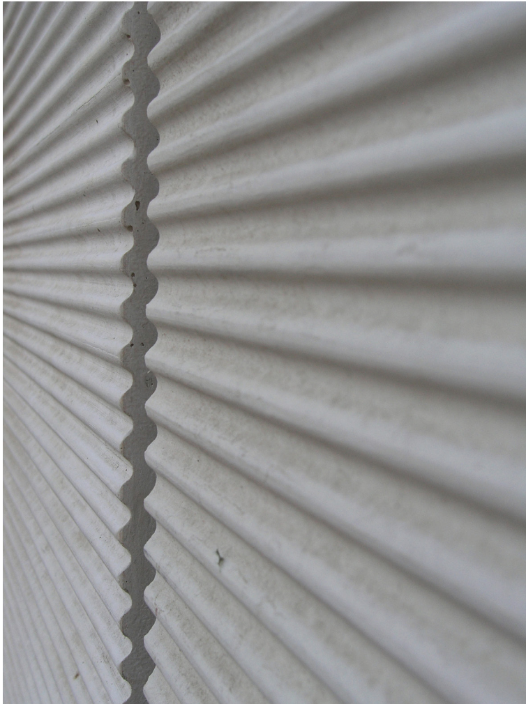
Figure 14 The facades in Gyldenrisparken were re-insulated and covered behind new fibre-concrete elements. They build on the original tectonics of the buildings, but creamy colouring and new profiling add new textural qualities and experiences to the buildings. Photo: Tegnestuen Vandkunsten.
