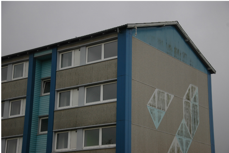
Figure 6 Ådalen in Struer after it was renovated in the early 1990s. The original facades have been hidden behind Steni coverings; colours have been added around entrances, and artworks adorn the end walls. Despite these ornamental effects, the rhythm and horizontal structure of the buildings have been preserved. Photo: Claus Bech-Danielsen.
